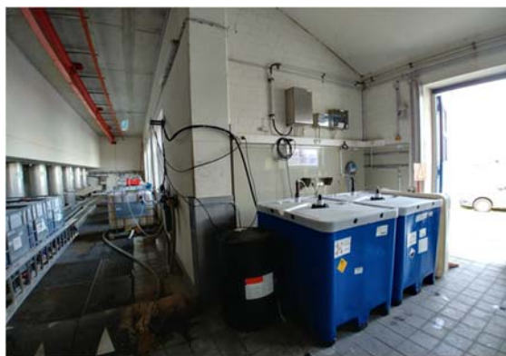
Chlorine dioxide pilot plant
