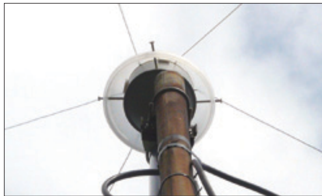
Figure 9 — Switch unit with dipole wires and weather protection cover placed on top of the supporting mast.
